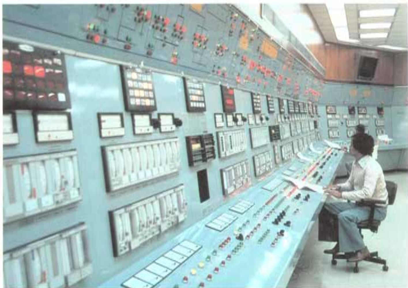
Abu Fontas Power Station
